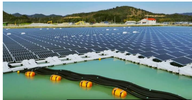
Fig. 15: Floating Solar Panels (Harrington, 2016)
