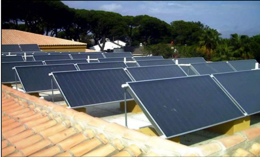
Fig.10: Rooftop Solar PV Panels (tilted)
